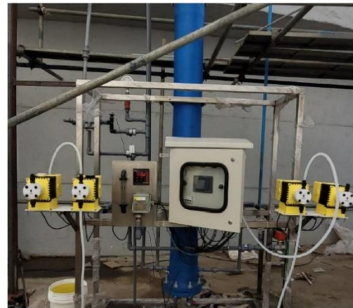
PureOx ClO 2 Generator - Installed at site
