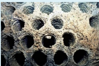
Above picture shows scaling in cooling tower.
